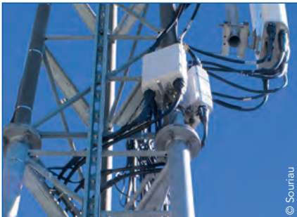
Cell Tower Distribution Box
